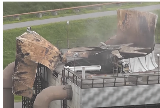
Preventable damage to a cooling tower.
